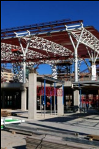
The International room at Calgary Airport's new 2 million sq. ft. terminal includes Customs areas for Canadian and U.S. border agencies. To meet the agencies' sound attenuation STC rating requirements cost-effectively, PABCO Gypsum QuietRock ES sound-deadening drywall is being installed.
