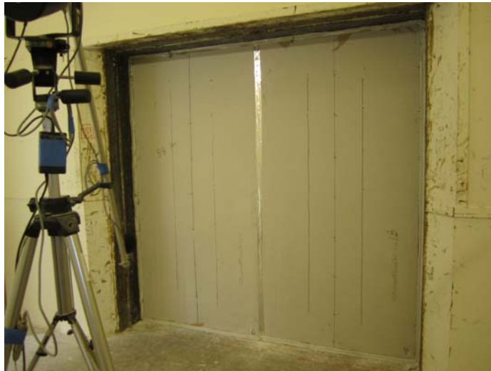
Figure 2: Source room side QuietRock ES sheeting installed and sealed in the specimen opening
